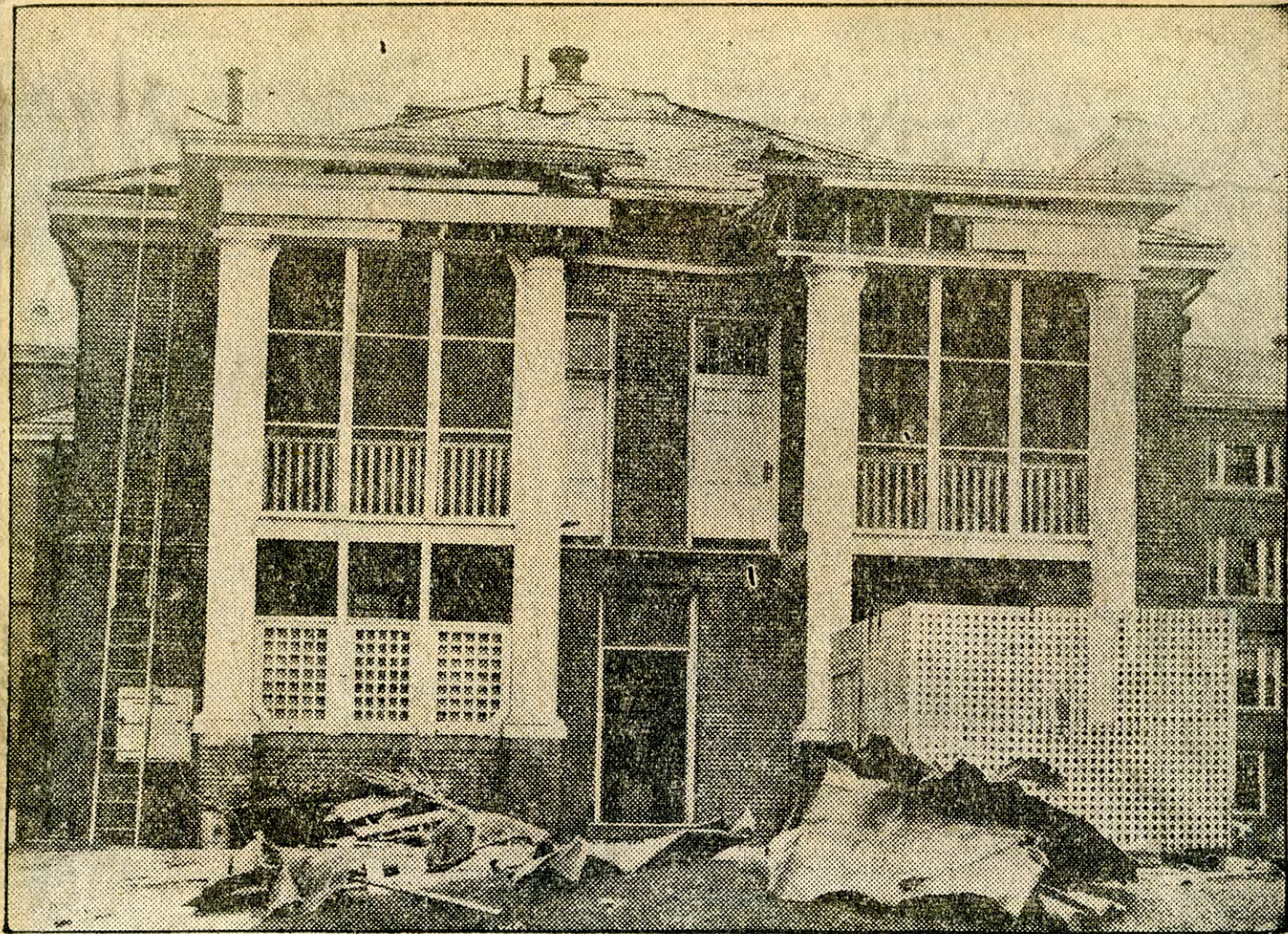
WHERE TWO GIRLS DIED AT NORTHFIELD: FRONT VIEW OF GOULD HALL AT NORTHFIELD seminary showing wreckage left by falling masonry which killed two students and injured others during Wednesday's hurricane.
