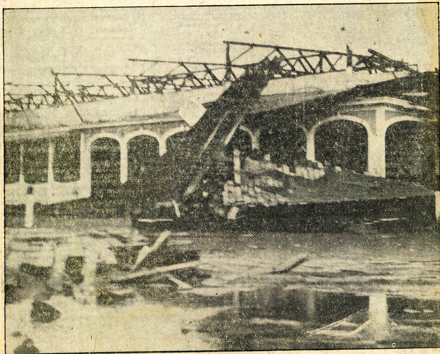
EXPOSITION GRANDSTAND ROOF GOES: THE WHOLE ROOF WAS BLOWN OFF AND HURLED to the ground below.
